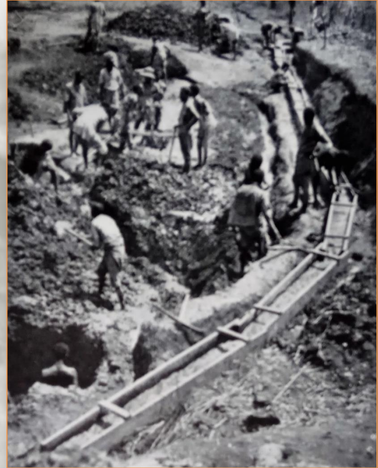
Construction of a water canal, presumably from the Birbir River to Tulu Kapi
